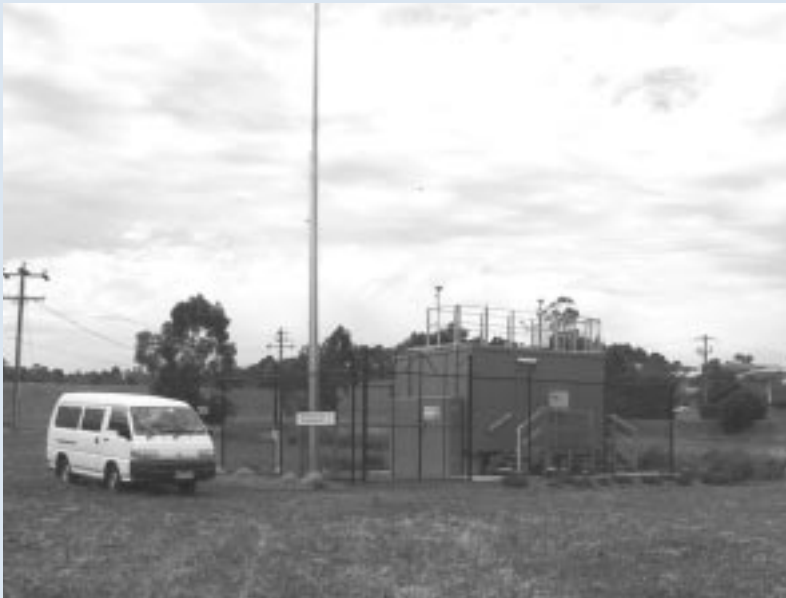
Melbourne's new Mooroolbark air monitoring station.
